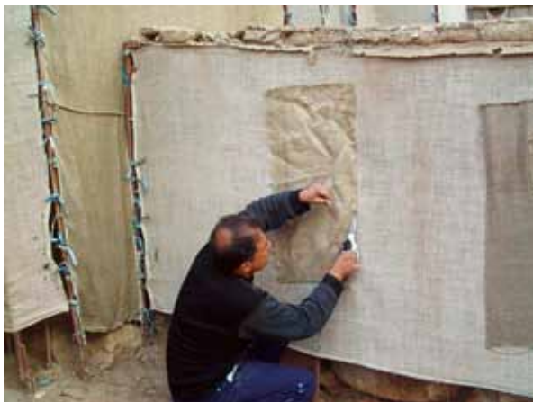
Figure 13. Patches on panels.
