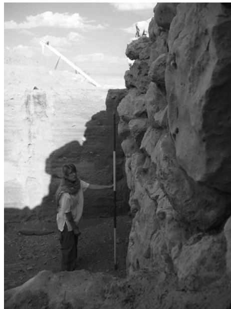
Fig. 3 The high revetment wall as a barrier with stadia rod emphasizing verticality
