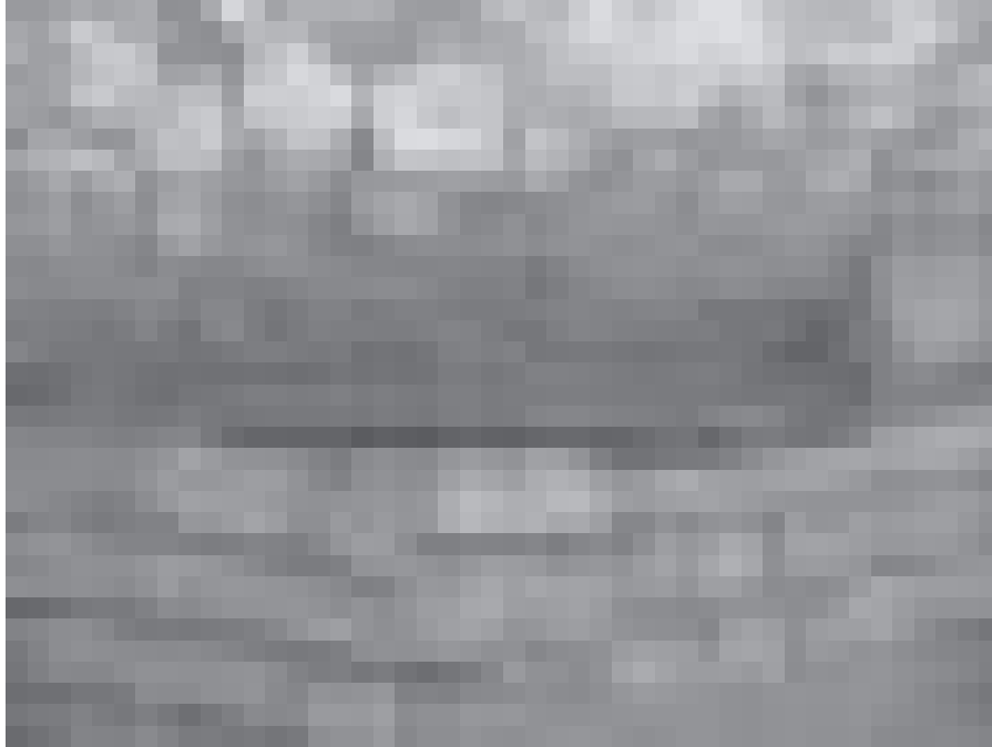
Fig. 10: Direct overhead of stone escarpment and revetment wall (photo by Federico A. Buccellati)
